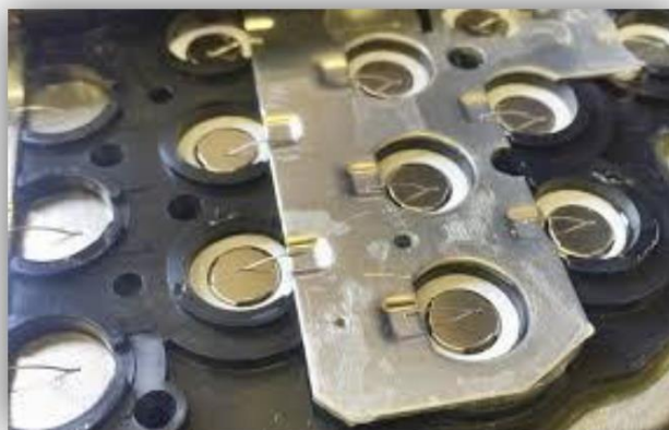
Cells Electrical connection to Bus Bar.
