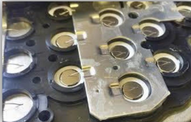
Cells Electrical connection to Bus Bar.
