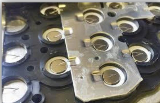
Cells Electrical connection to Bus Bar.
