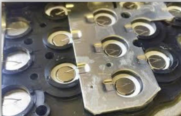
Cells Electrical connection to Bus Bar.
